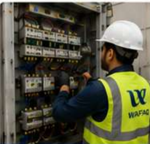
CONTROL & RELAY PANELS
