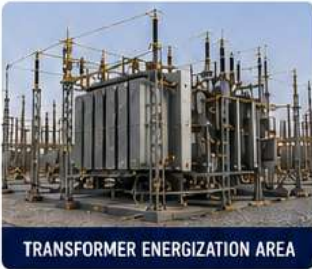
COMPLETED SUBSTATION YARD
